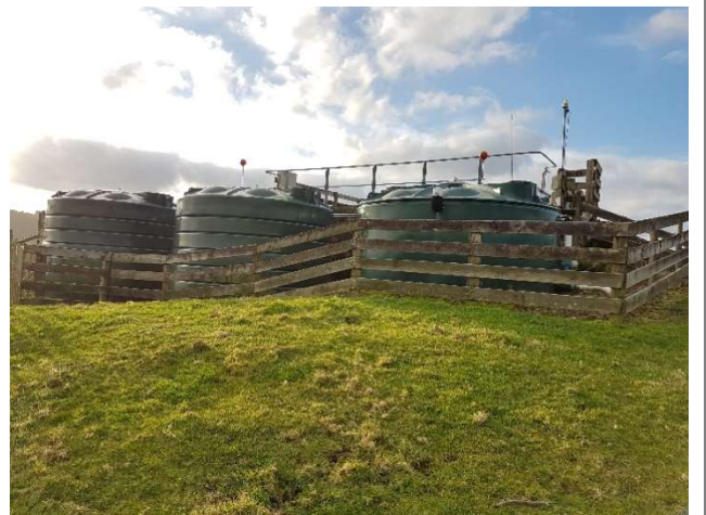
Figure 7. Treated water reservoirs
