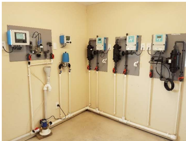
Figure 6. Online monitoring equipment
